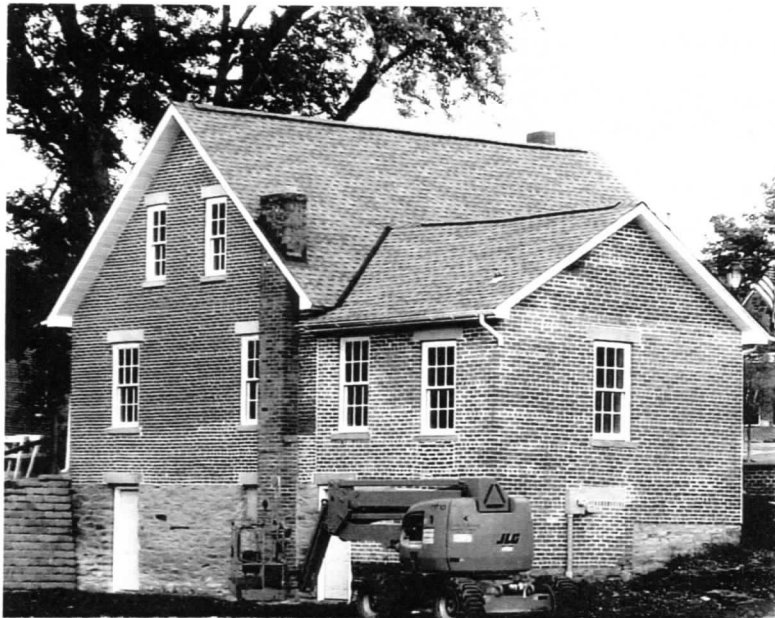
South and west sides of the newly restored Phelps House in the center of New Albany, Ohio
